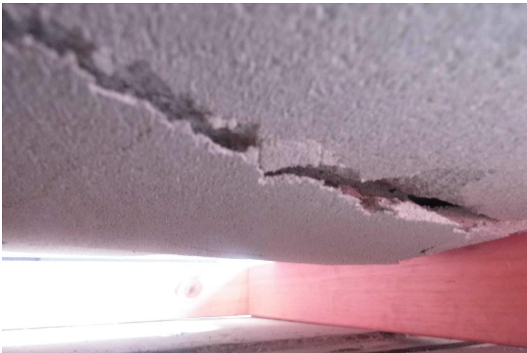
Figure 11 Typical failure pattern on the underside of the panel (100 mm x 100 mm foot)
