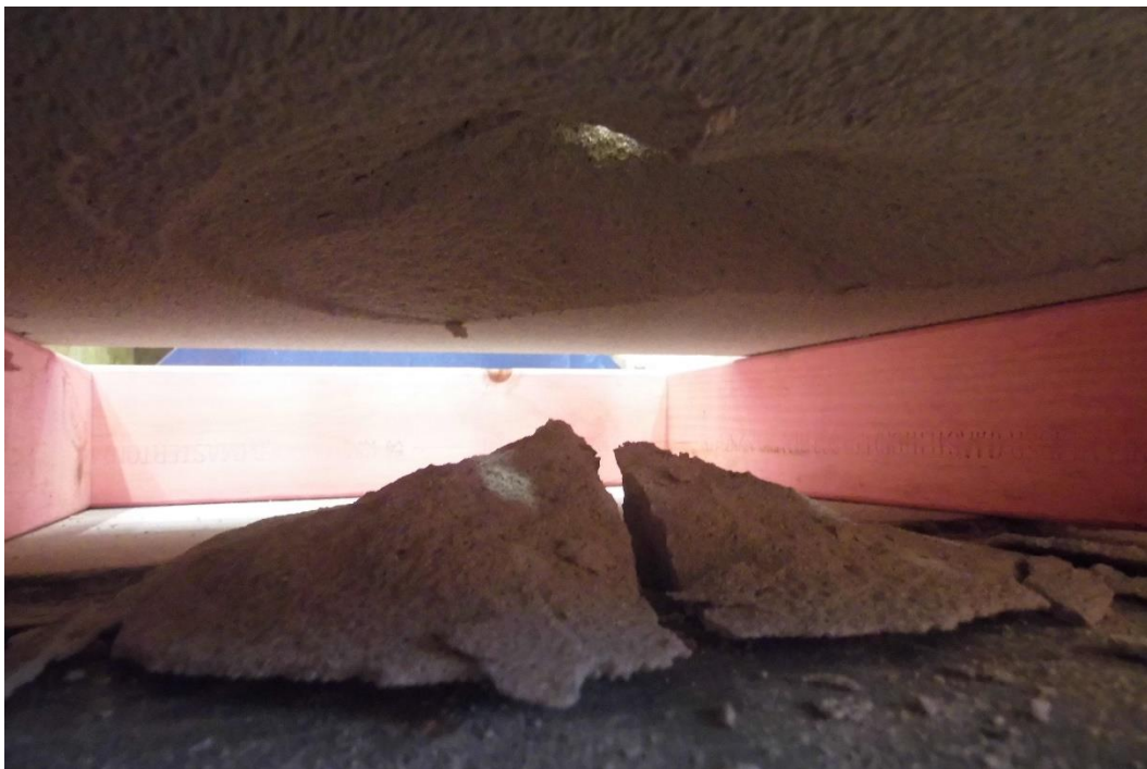
Figure 9 Typical view of the underside of the panel after the 20 mm foot punched through
