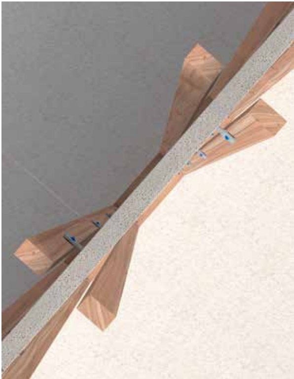
Image 10 – Brackets shown on different studs on opposite walls
