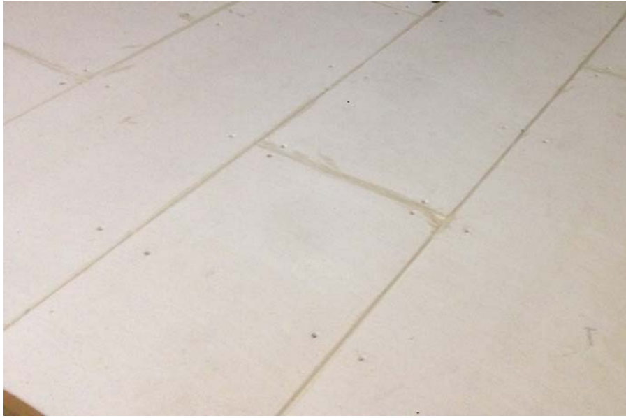
Figure 3: Rockcote floor surface showing screw-fixings and sealant in joints
