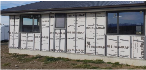
Figure 5: Unacceptable installation without closure strip at bottom?? If the cavity closer is installed
