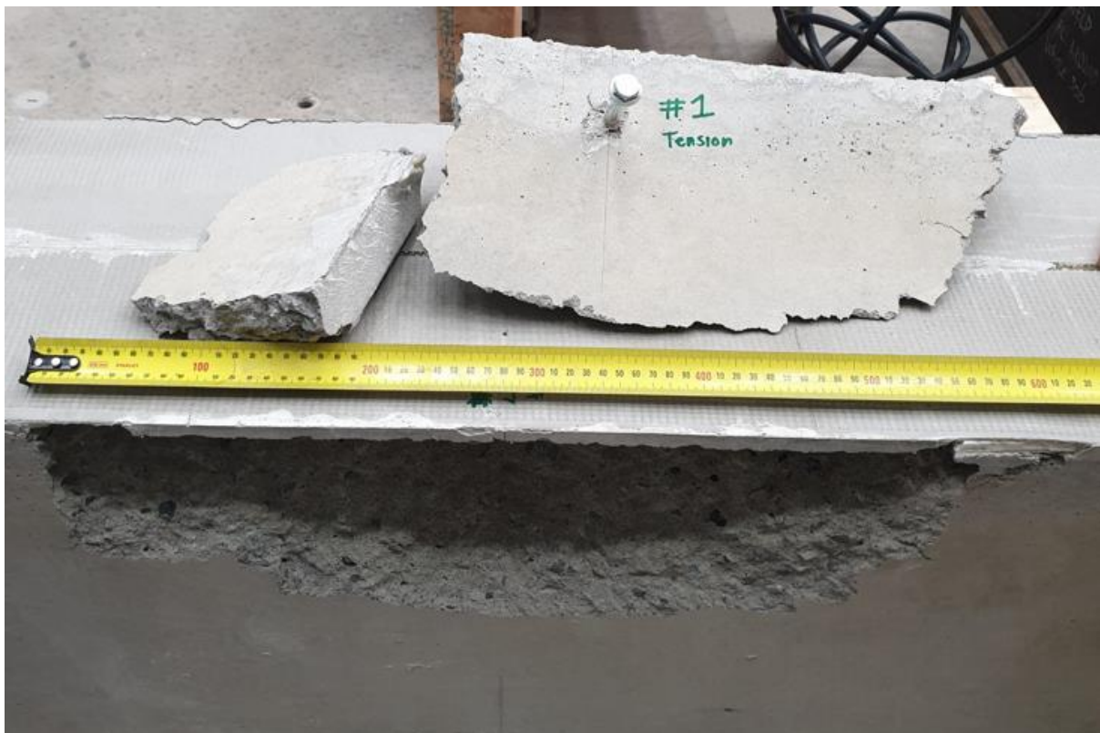
Figure 9. General failure from tension loading.
