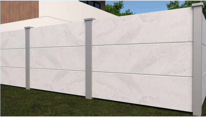
A rebate has been formed between the panels prior to applying the finish coats of plaster and paint.
